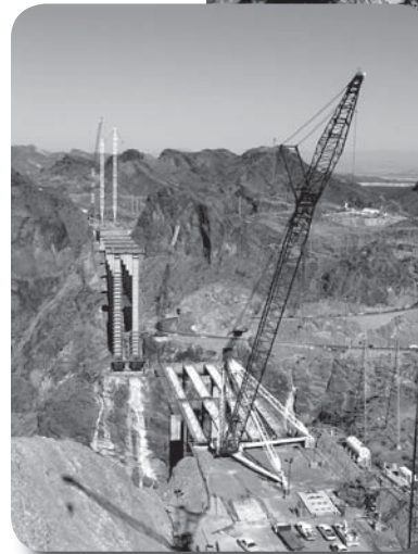
Pictured left is the structure in which our product is being utilized to construct the bridge. (Photo provided by F&M Mafco)
