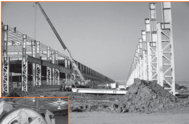
Pictured above is the frame of the one million square foot manufacturing facility in Wuhan, China.
